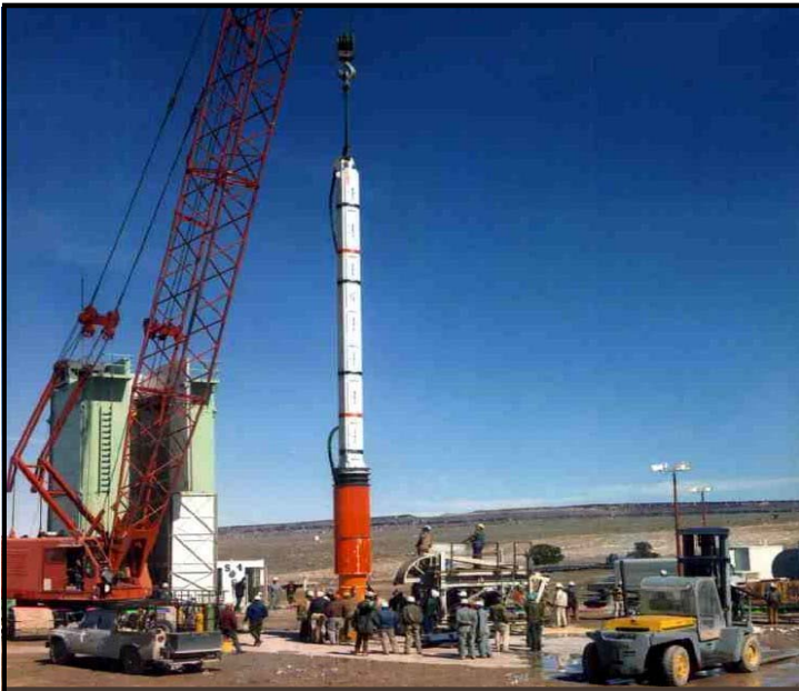
A "DEEP-SHAFT" TEST DEVICE IS BEING SET UP AT THE PHYUTE-MESA AREA OF THE NEVADA TEST SITE
