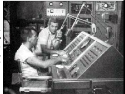
Back in the Control Room – Now What ??
